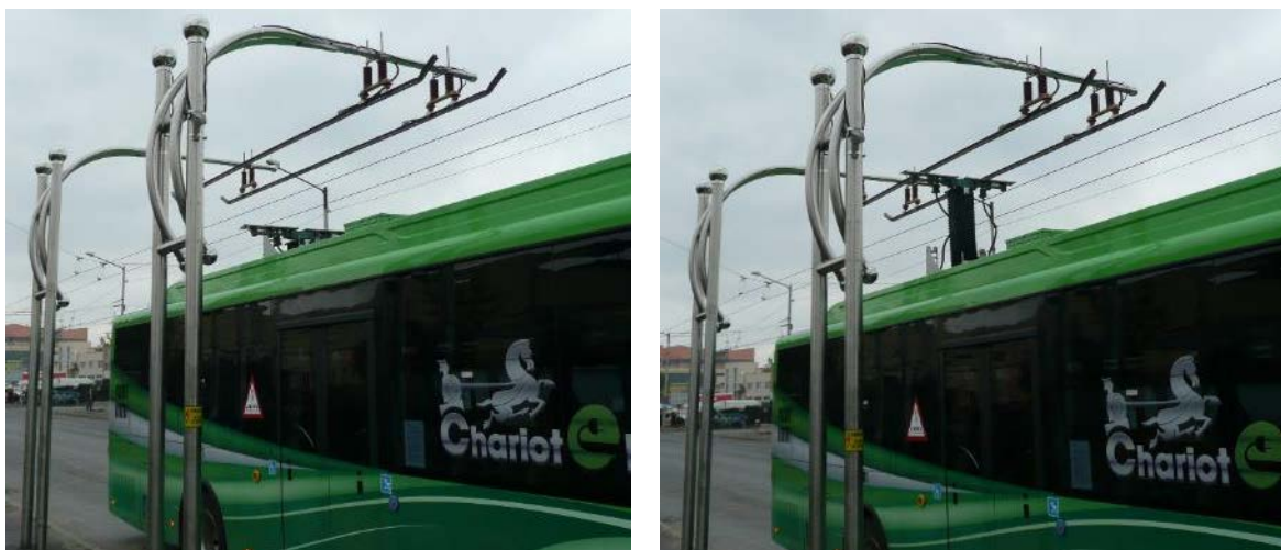
Figure 2-2 Pantograph Docking at the Charging Stations
