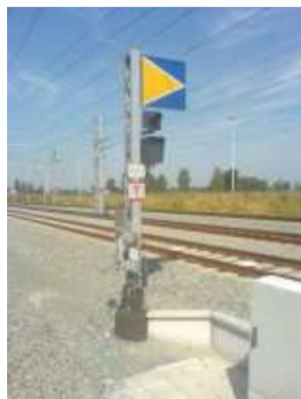
Figure 26: ERTMS/ETCS Marker boards
