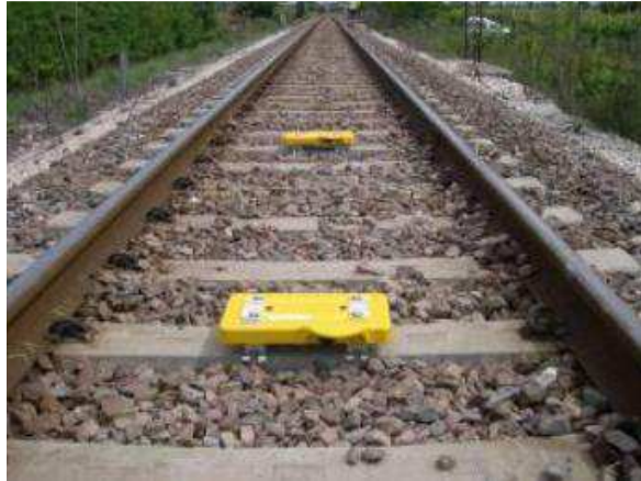
Figure 25: Eurobalises on a railway track
