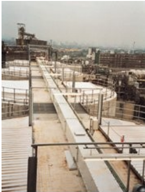
Typical over-silo conveyor
