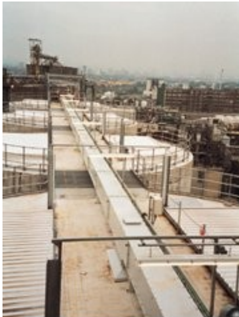
Typical over-silo conveyor
